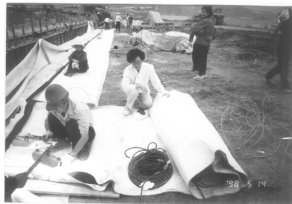
图4 安装好土工膜应变计的防渗土工膜与现场土工膜连结 Fig.4 Connecting the geomembrane with strain gauges to the field waterproof geomembrane
