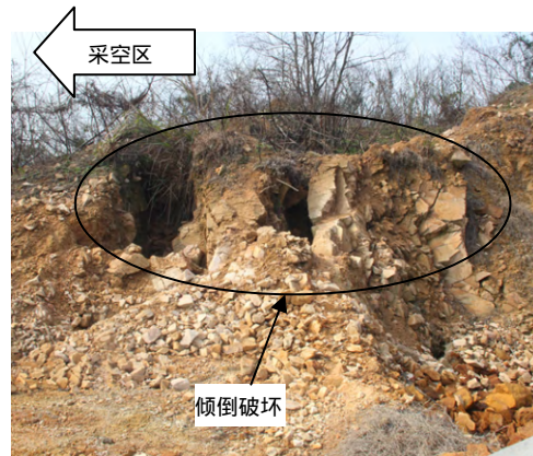
图 27 采空区边缘岩体倾倒破坏 Fig.27 Rock mass toppling failure around goaf
