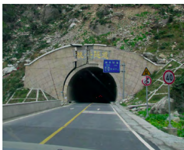
图6 桃关隧道入口端墙开裂 Fig.6 The end wall cracking at the entrance of Taoguan tunnel
