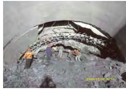
图7 龙溪隧道垮塌 Fig.7 The collapse in Longxi tunnel
