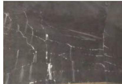
图8 酒家垭隧道衬砌开裂、渗水 Fig.8 Lining crack and water seepage in Jiujiaya tunnel
