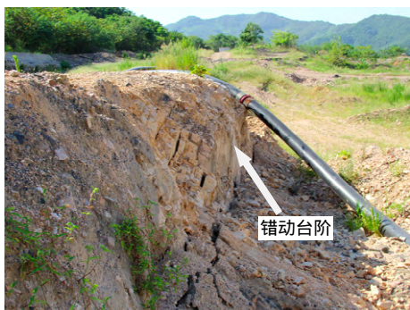
图 5 粉矿堆场处的错动台阶 Fig.5 Dislocation steps in the fines yard
