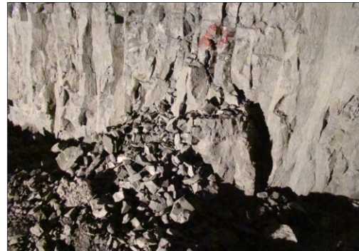
图 6 柱状节理岩体沿节理面滑移 Fig.6 Joint slip of columnar jointed rock mass
