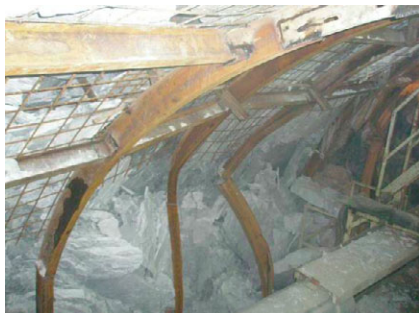
图 2 锦屏二级水电站施工排水洞岩爆导致钢拱架扭曲 Fig.2 Steel arch distortion by rock burst in Jinping II hydropower station drainage tunnel
