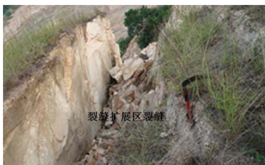
图 18 粉矿堆场附近地表裂缝 Fig.18 Surface cracks of yard of fine ore
