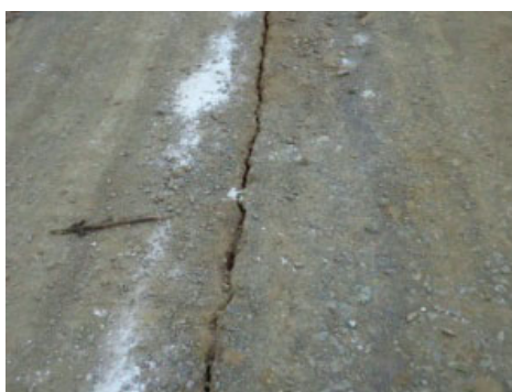
图3 渠坡后缘裂隙 Fig.3 Crack at the crown of slope
