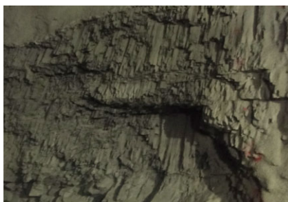
(b) 边墙柱体松动垮塌
