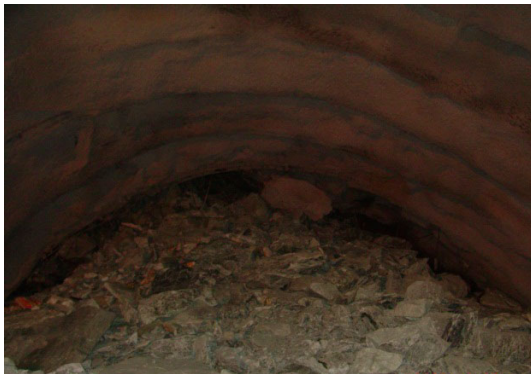
图1 绿泥石片岩洞段塌方 Fig.1 Collapse in chlorite schist section
