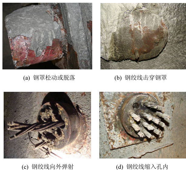
图 3 对穿预应力锚索失效的现场破坏形式 Fig.3 Field failure formats of prestressed thru-anchor cable
