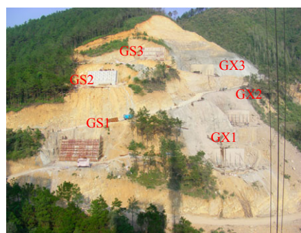
图 14 广州岸预应力锚碇系统 Fig.14 Anchorage system on Guangzhou bank slope
