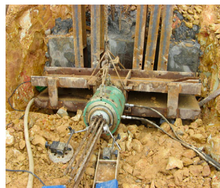
图 4 GS2 锚碇处的现场拉锚试验 Fig.4 Anchor test of prestressed cable in GS2 anchorage
