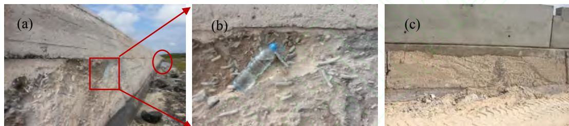
Fig.1 Corrosion characteristics of coral aggregate concrete
