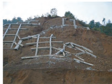
图1 高速公路沿线边坡破坏图 Fig. 1 Destruction of slope along the highway
