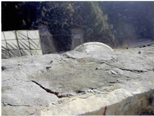
图 1 泰山沟隧道进口边坡左洞拱顶变形迹象 Fig. 1 Deformation features of the left vault on the entrance slope of Taishangou Tunnel
