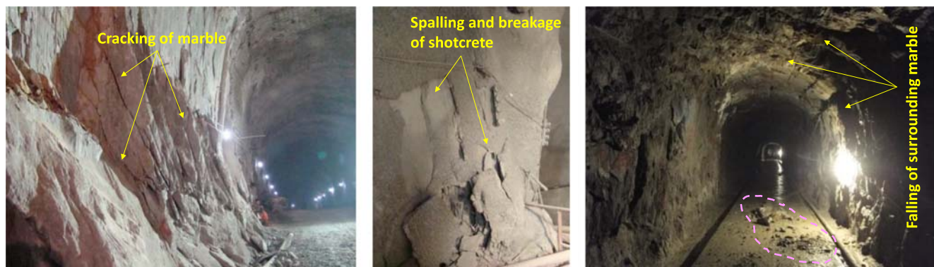
Fig. 1 Typical time-dependent failures of Jinping marble
