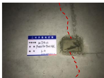
Figure 2. Cracking of the lining structure.
