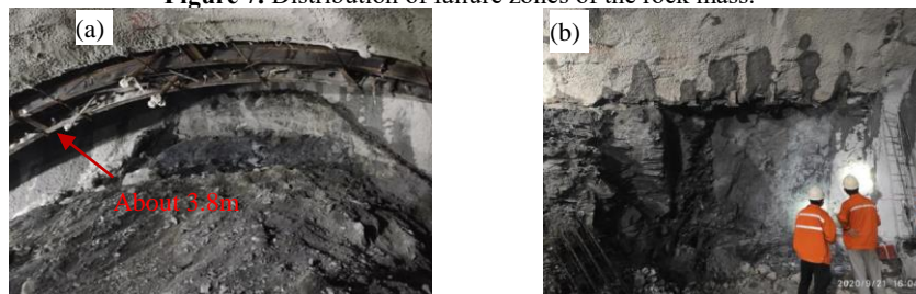
Figure 8. Actual collapses during tunnel excavation (a: collapse on the left arch; b: collapse on the right-side wall).
