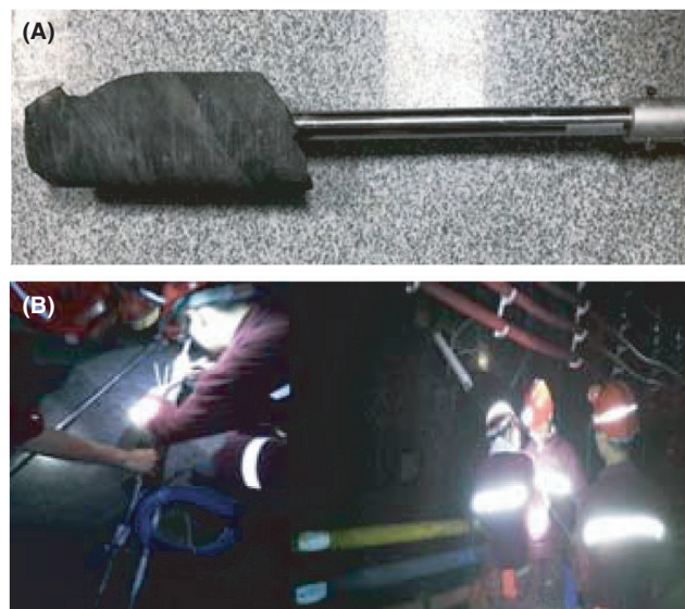
FIGURE 4 The core with sensor by overcoring test (A) and on-site installation work (B)
