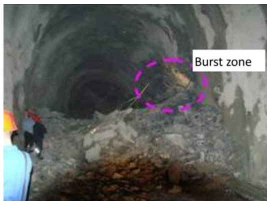
Fig. 5 The extremely intense rockburst at BK9+516-538 in the auxiliary tunnel #B
