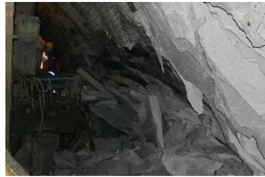
Fig. 29 The intensive rockburst on the north sidewall of the headrace tunnel #3 during the full-face TBM excavation
