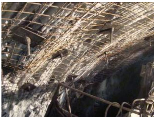
Fig. 25 The layered fracture in the surrounding rock mass of the headrace tunnel #3 during the full-face TBM excavation (Zhang et al. 2011b)
