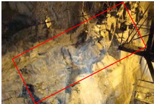
Fig. 28 The collapse of the fractured rock mass on the south sidewall of the headrace tunnel #3 during the TBM excavation
