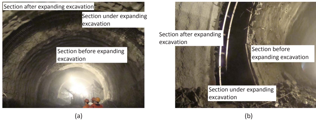
Fig. 5. Expanding excavation scene in the chlorite schist extrusion deformation section: (a) arch crown; (b) skewback.
