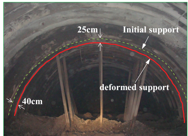
Figure 6. Excess of clearance limit after installation of the primary lining.
